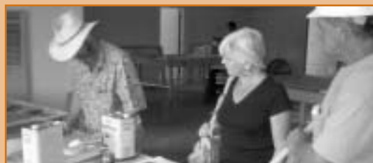
AJHS board member Susan Shaffer Nahmias watches as carpenters restore historic windows, July 14th
